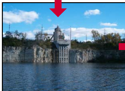
West lobe pump station. West lobe is pumped out first.
