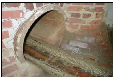
Likely illicit discharge with bacterial growth from raw sewage outfall. (Photo courtesy of the Center for Watershed Protection)
